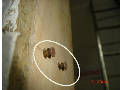
Figure 10. Nail withdrawal between LVL structural members
