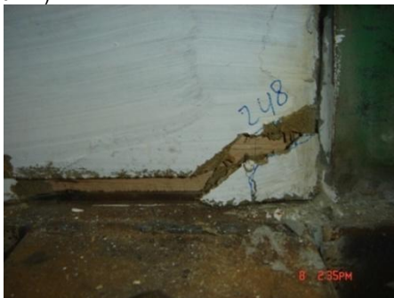
Figure 11. Part of the CFB panels were broken because of the deformation order sliding wall panels
